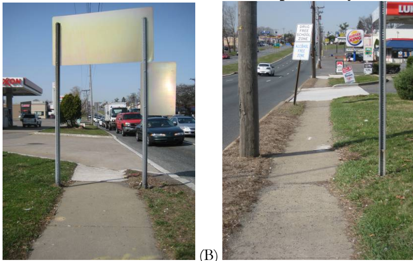
Route 22 Sidewalk Condition West of Roseberry St & Route 22 Intersection: (A) Southern Side (B) Northern Side
