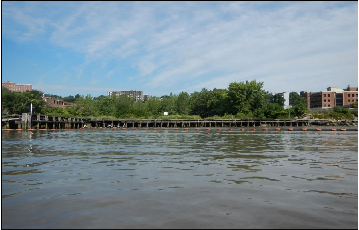
Photo No. 1 – Deteriorated timber platform along shoreline. Shallow water approach.
