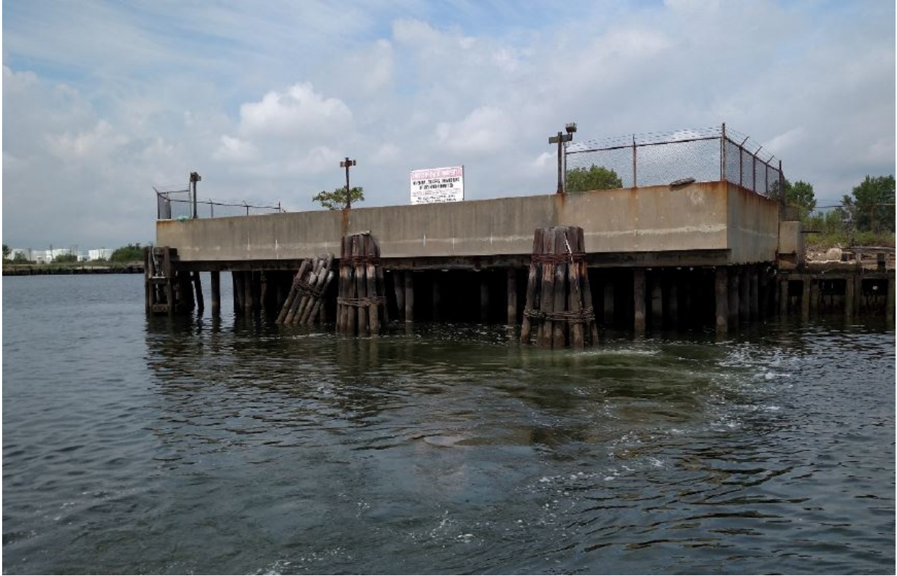
Photo 1 – Pipe pile supported concrete platform and timber dolphins at southeast corner of property.
