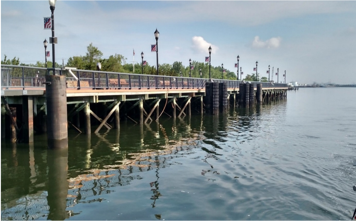
Photo 1 – New timber pier with breasting panels and hardware for mid-sized vessel berthing capabilities.
