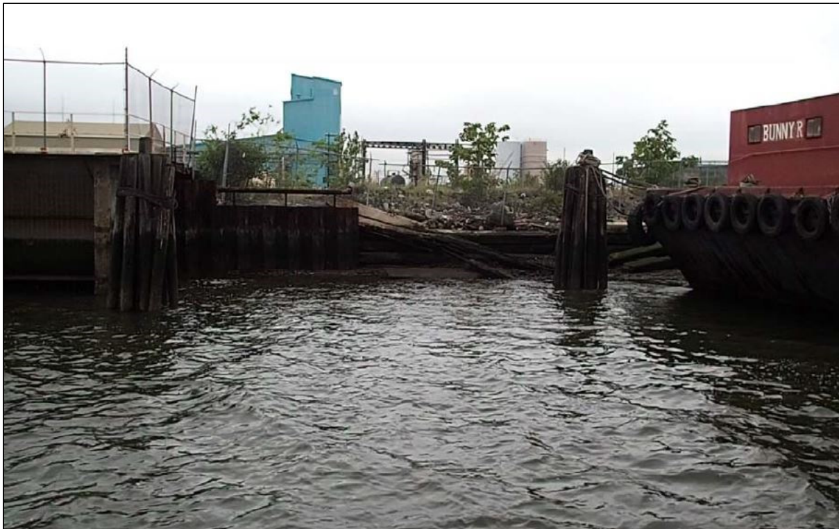
Photo No. 2 – South end of berth. Abandoned intake structure to left, barge in berth to right.
