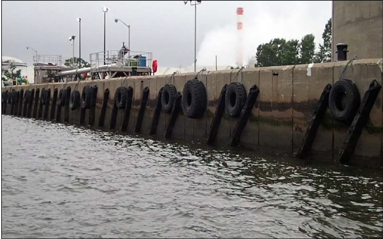
Photo No. 1 – Concrete fascia that provides the berthing area. Rubber breasting panels in place.
