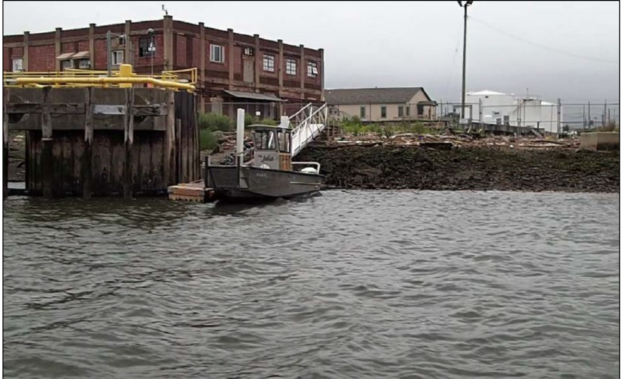
Photo No. 1 – Small boat landing at the north end of the site replaced a collapsed timber platform.
