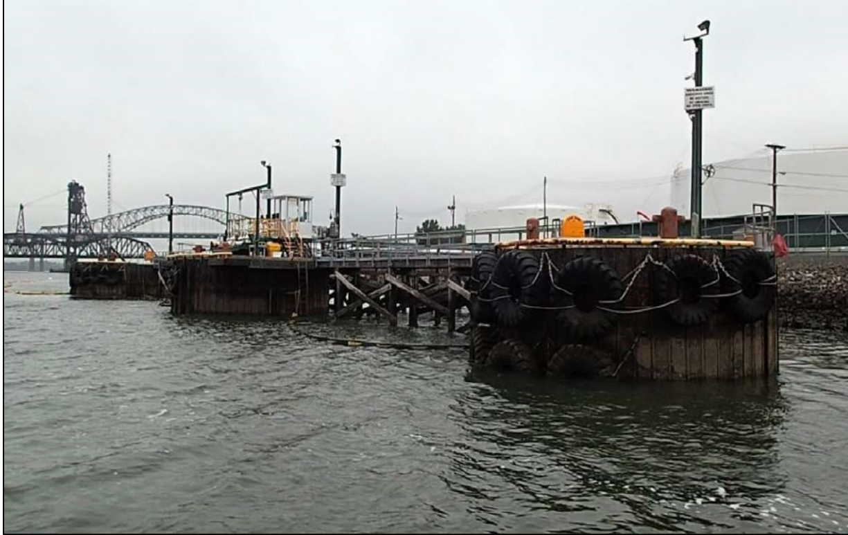
Photo No. 1 – Three steel sheet pile cell berth. Center cell is the loading platform.
