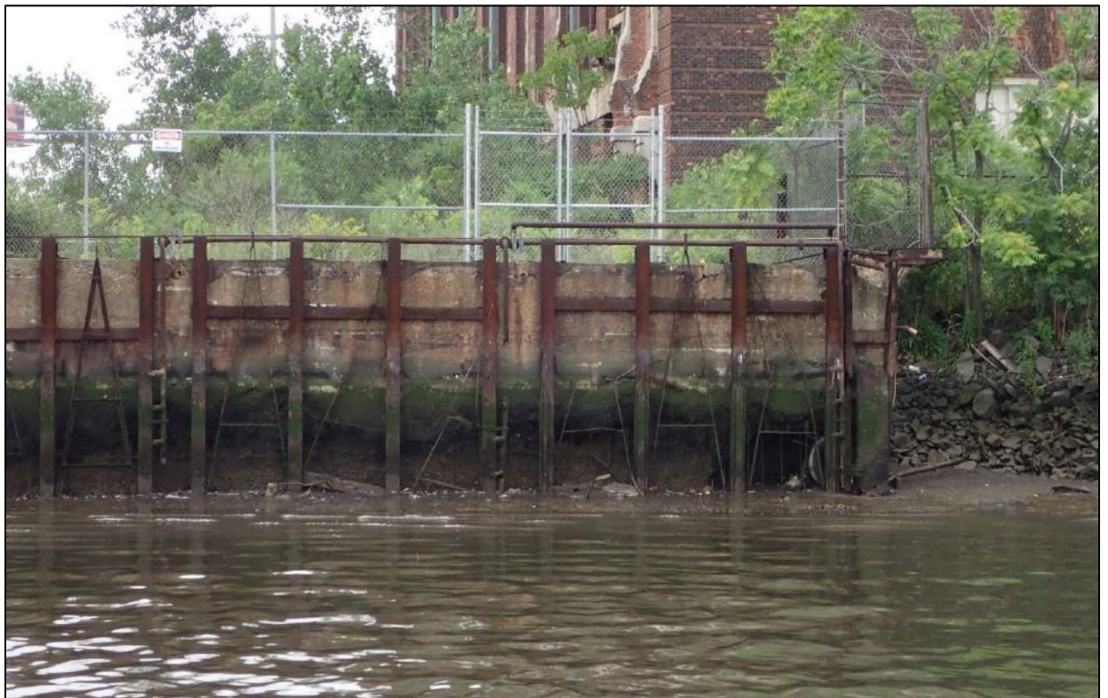
Photo No. 2 – Undermined concrete bulkhead at the north end of the site.
