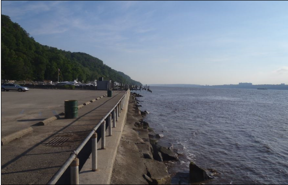
Photo No. 1 – View to north of concrete and stone seawall. Note marina to the north.
