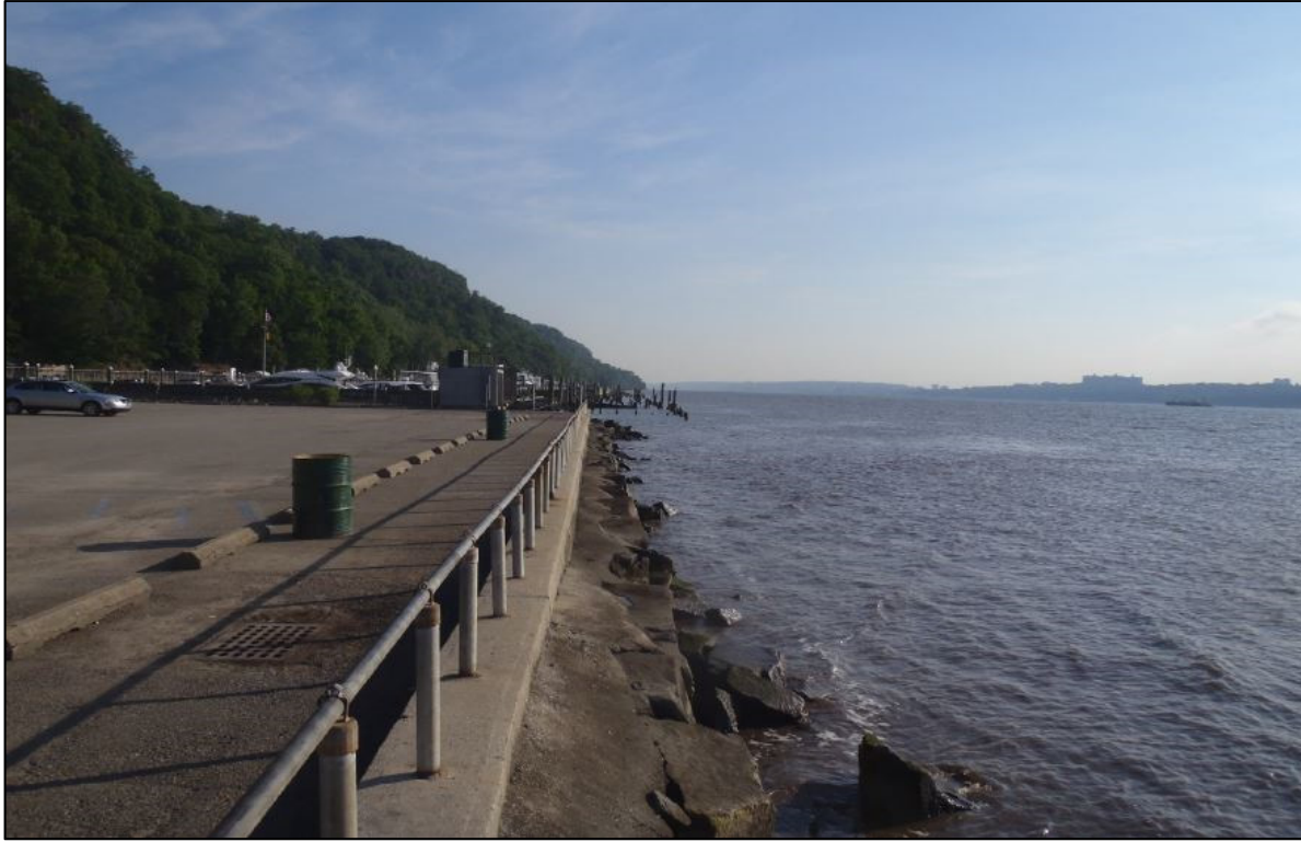
Englewood Cliffs – View to North of Concrete and Stone Seawall; Note Marina to the North
