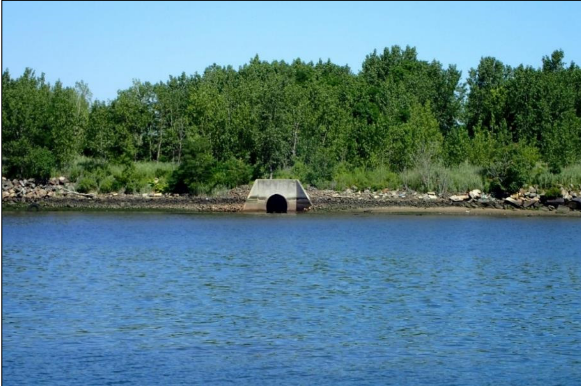
Elizabeth Waterfront – Large Diameter Outfall Located Along Shoreline of Southern Portion of Site
