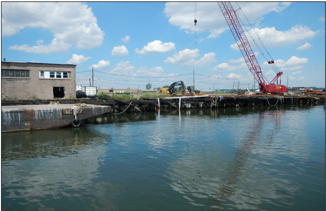
Photo 2 – East end of abandoned wharf structure. Piles and caps remain. Area is utilized by contractor.
