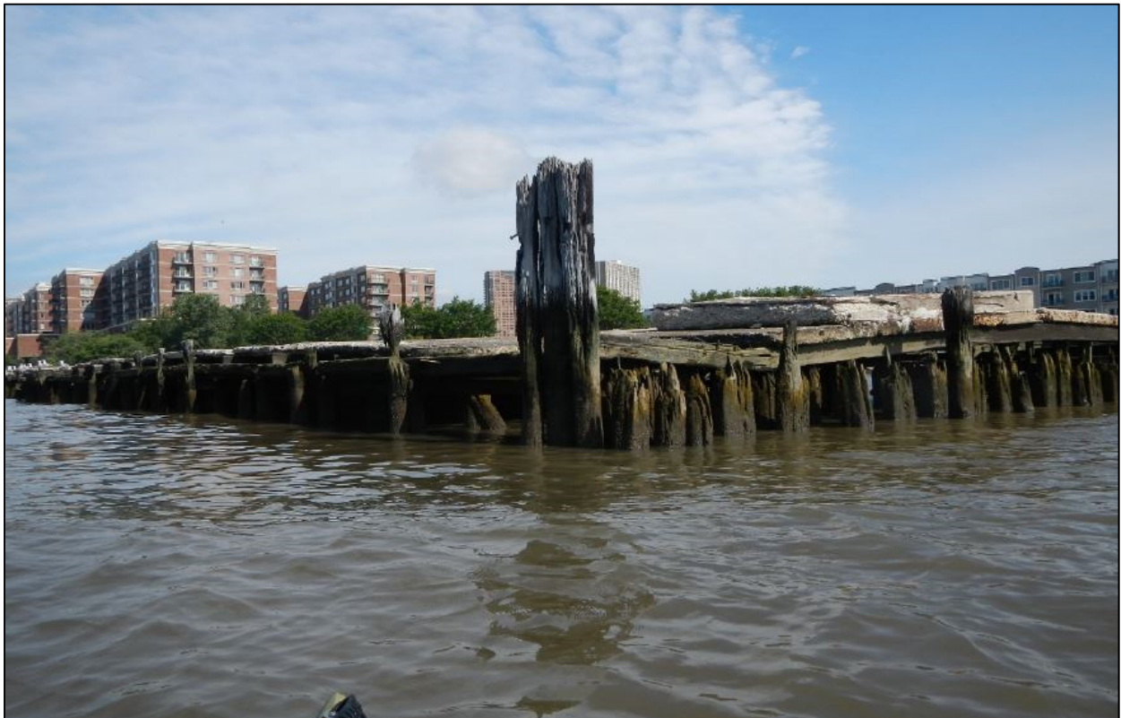
Photo No. 2 – Collapsing timber pier and concrete deck at north side of the site.
