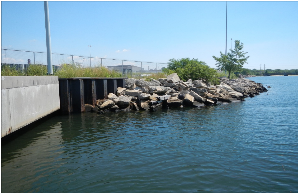
Photo 2 – Sheet pile return precedes rip rap shore protection to the east of the wharf.
