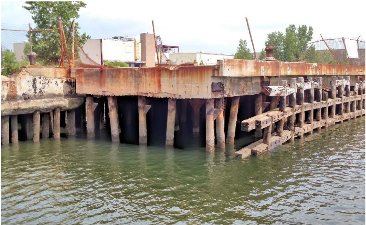
Photo 2 – Pipe pile supported wharf with timber fender and mooring hardware at eastern exposure.
