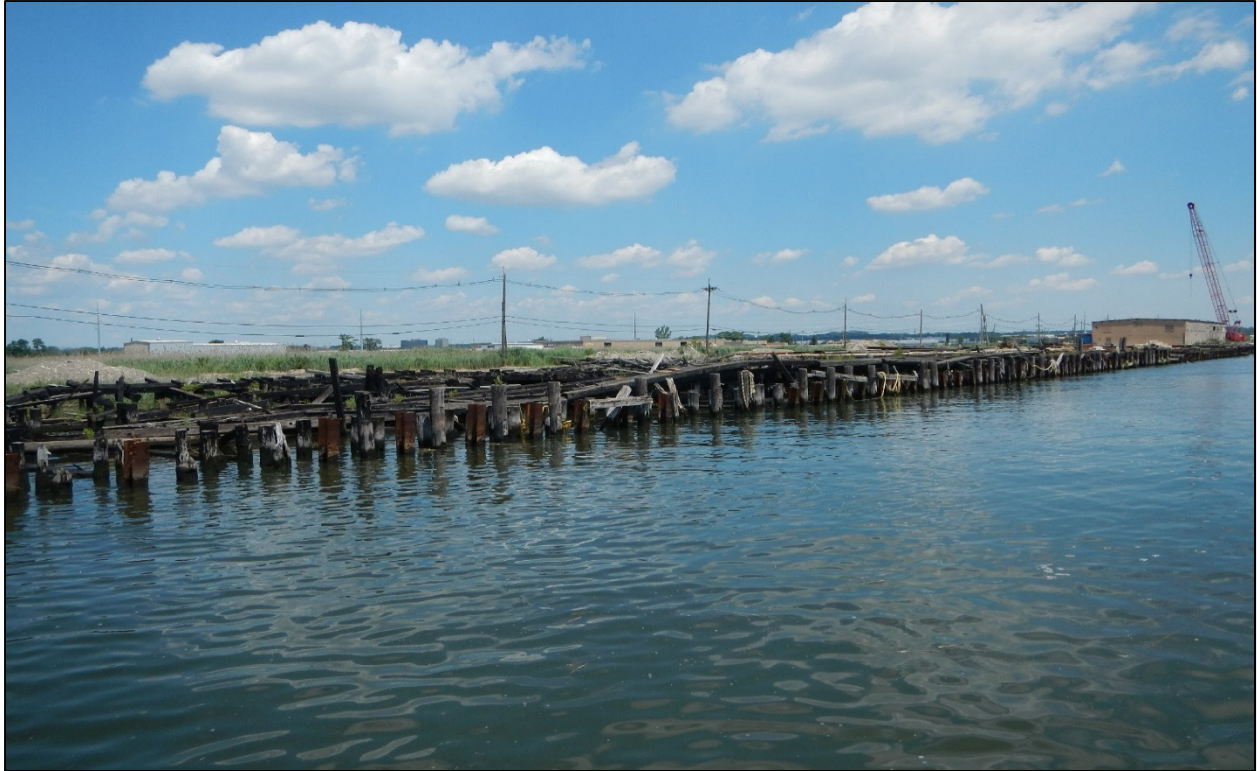
Photo 1 – West end of abandoned wharf structure. Piles and partial caps remain.
