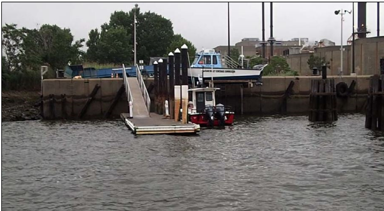
Photo No. 2 – Small boat landing and timber dolphins located at the south end of the berth.
