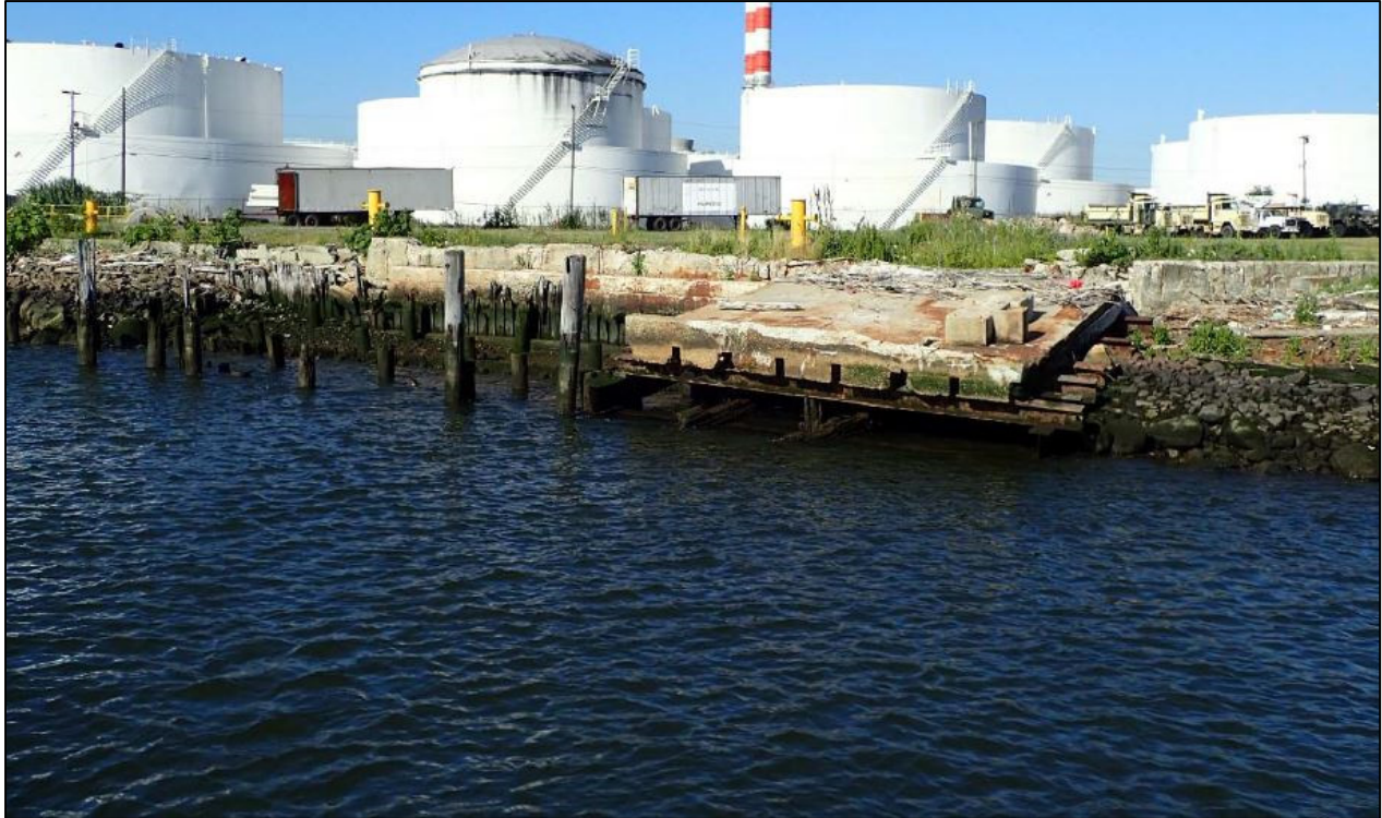
Photo No. 1 – Collapsed timber platform with concrete deck.
